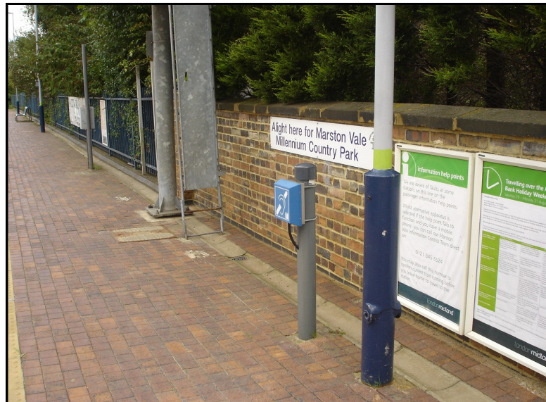
Post mounted Omni-T150, Millbrook Station, Marston Vale (London Midland)
